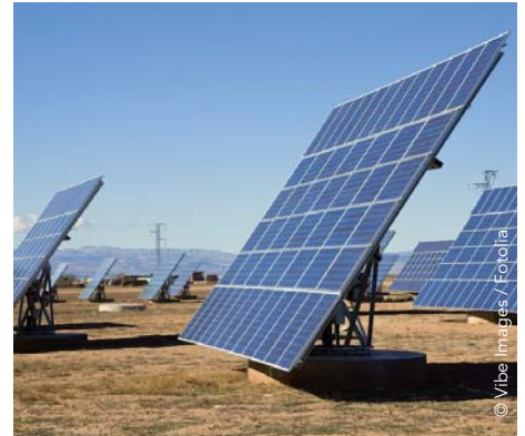
Control Unit / Solar
